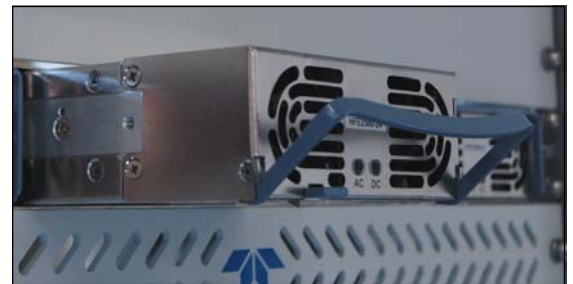
Power Supply Module in Chassis
